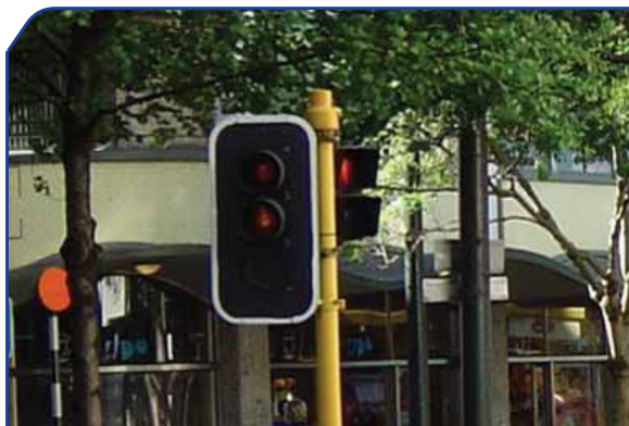
Figure 9 : Non-complying two-aspect display (green missing).
